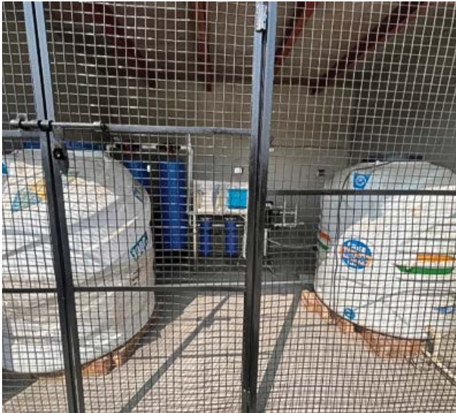
Figure 3: Water Purifier and Water Tanks
